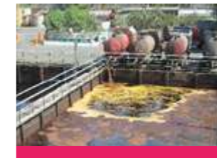
Common effluent treatment plant
